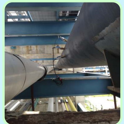
Power Plant Circulation Water
