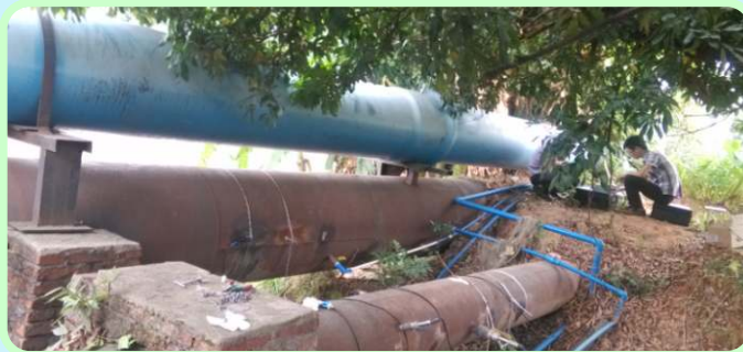
DN800 Water Supply
